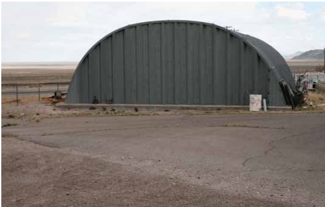
General rear view of the subject 2,280± square foot Quonset hut looking southeasterly
